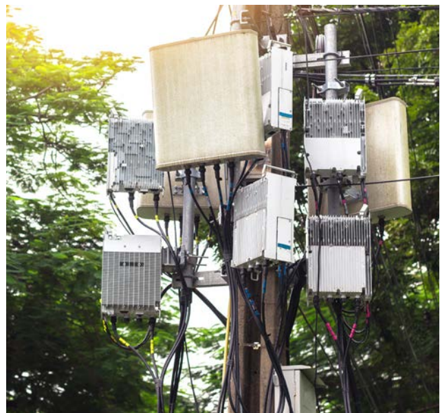
Wireless broadband infrastructure (Photo credit: Shutterstock)
